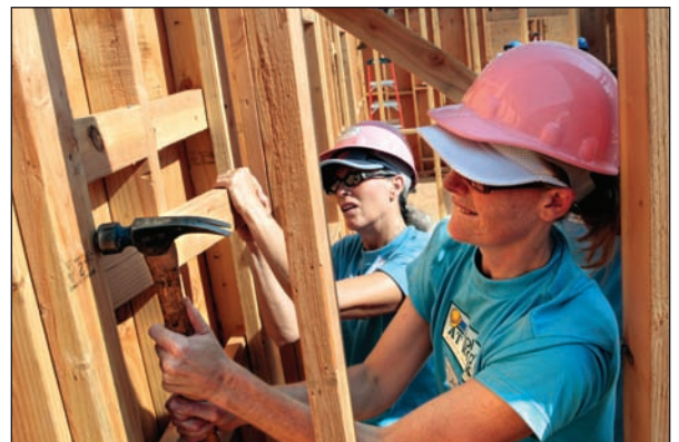
From left to right: Roland DGA Corporation employees Cindy Cao and Dede Logemann work together to reinforce an interior wall.
